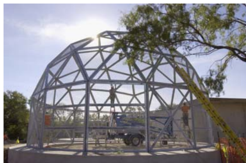
Construction workers put finishing touches on long-term chimpanzee housing. The housing is designed to allow chimpanzees to climb and rest in high places, as they do in the wild.
